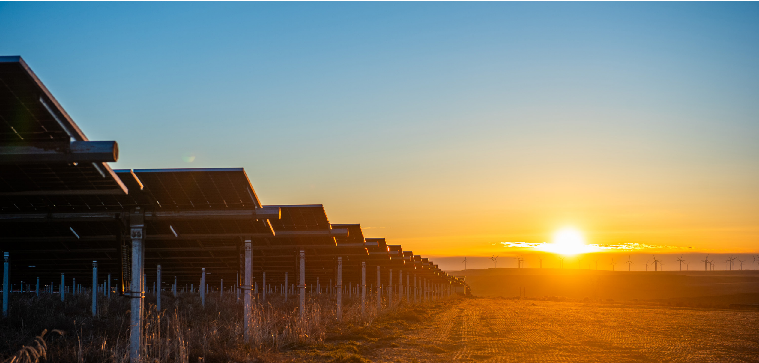
Black Mesa solar facility, Elmore County, Idaho
